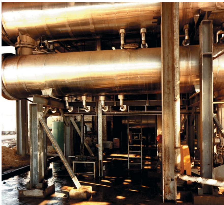
A tube digester, which is often used in nonwood fiber pulping.
